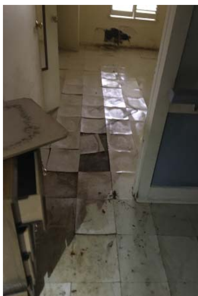
Tile Damage Due to Water Penetration
