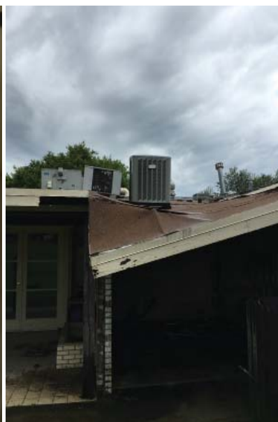
Failure of Roof Structure
