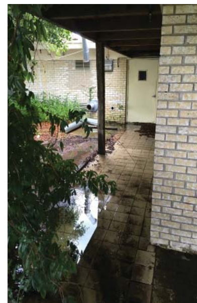
Example of Additional Water Drainage Issues at Site
